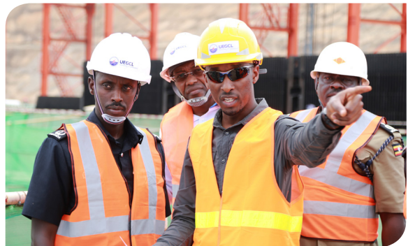
Albert Byaruhanga Musoke - Project Manager, UEGCL explains the project progress to Major General Steven Sabiiti Muzeyi - Deputy Inspector General of Police of the Uganda Police Force (R) during a site inspection at Karuma HPP on 12th February, 2019
