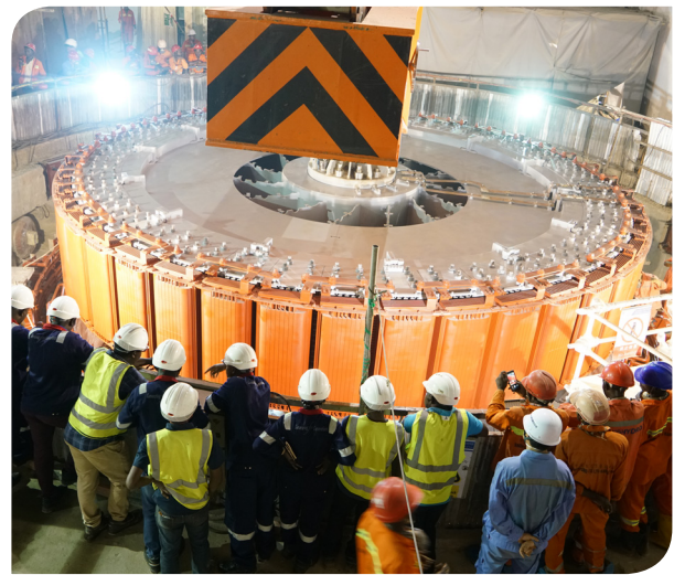
The last of 6 rotors for the 600MW Karuma HPP lifted and lowered into pit on 30th September, 2019.
