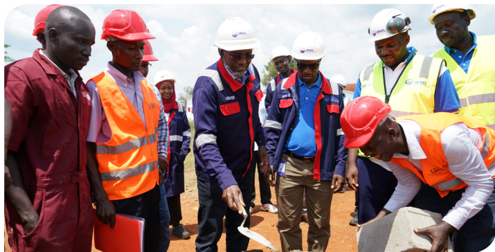
Dr. Eng. Harrison Mutikanga - CEO, UEGCL (C) lays the foundation stone for the Isimba HPS employers camp as part of the celebrations to mark 183 days of 183MW Isimba HPS.
