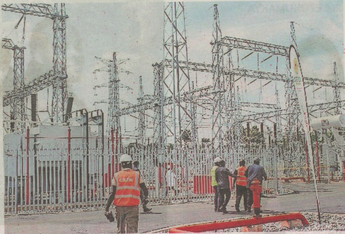
Technicians at the Nebbi power substation. A review of quarterly operations and maintenance reports shows mixed performance across major hydropower stations. PHOTO/FELIX WAROM OKELLO
